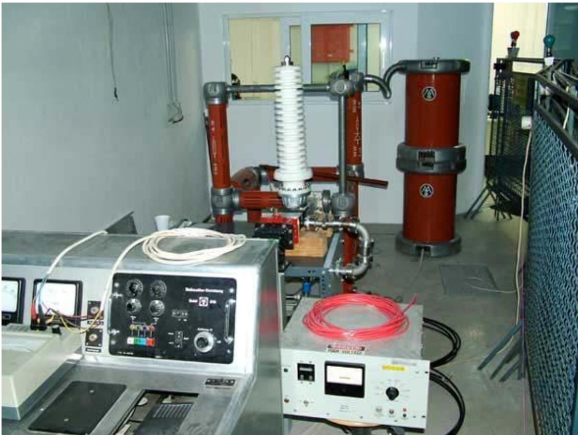
Fig. 6.13: Experimental Device with Impulse Generator VDE-b.
